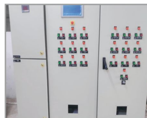
MCC cum PLC Panel
