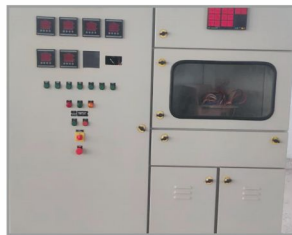
Governor Turbine Panel
